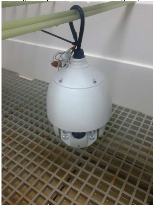
Fig.4 sample1#(during outdoor corrosion test)
